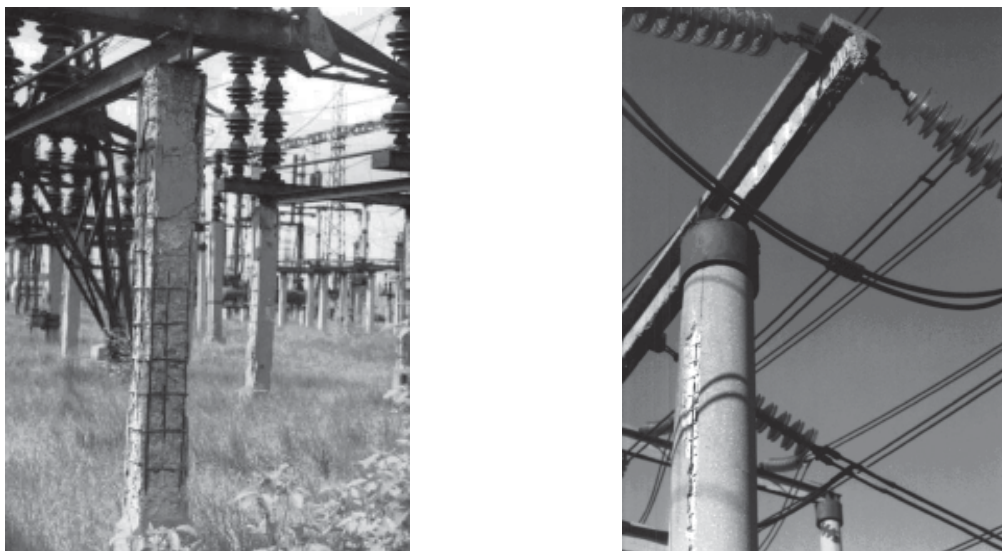
Fig. 6. Damages of column bases for outdoor switchgears.
