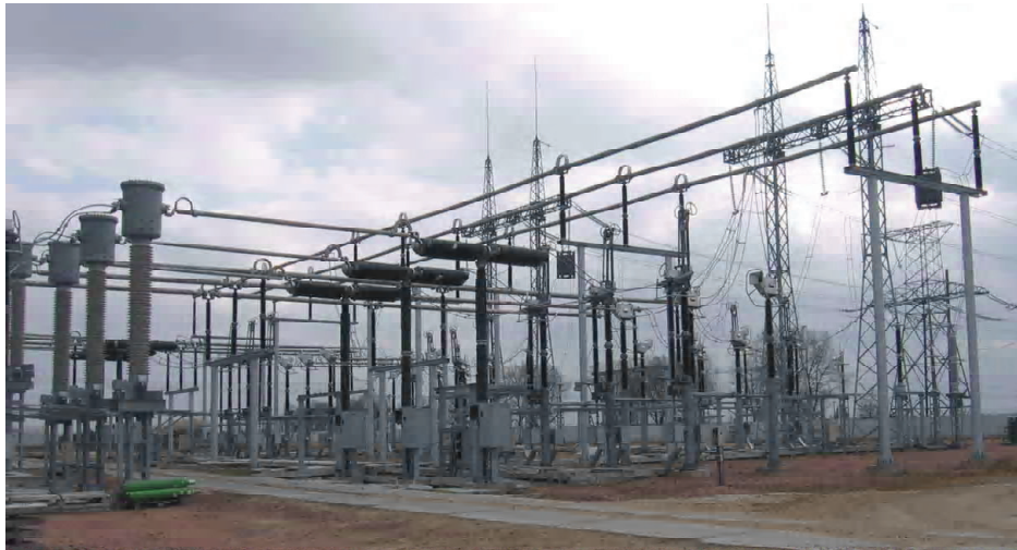
Figure 1. Rigid buses constructions of «Kievskaya» electric substation.
