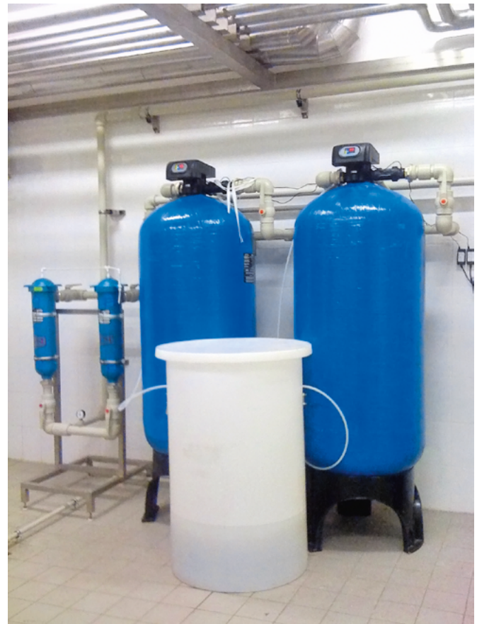
Figure 8. Water treatment station for a boiler room
